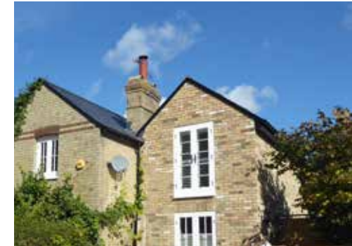
Figure 100: Visible satellite dishes and disproportionate modern windows distract from the appearance of buildings which otherwise contribute positively to the Conservation Area
