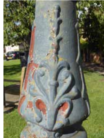
Figure 101: Street lamp requiring repainting, Little Green
