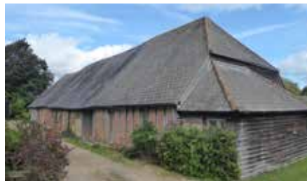
Figure 64: The barn at Rectory Farm, as seen from Shillington Road. View 4 on the map
