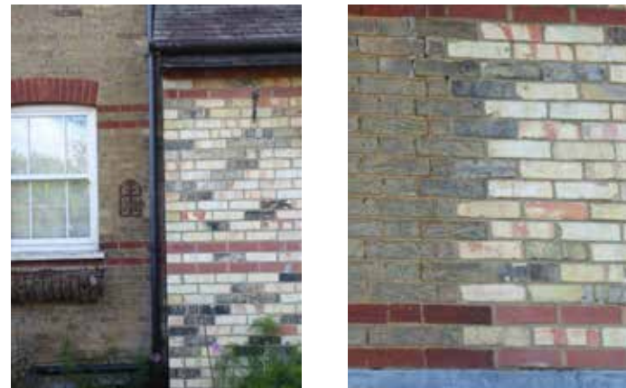
Figure 106: Poorly matched, bright modern brick, can contrast poorly next to original buildings if not well considered
