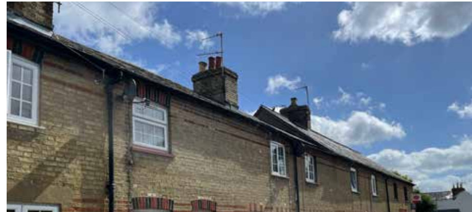
Figure 105: Example of a terrace where the replacement of windows diminishes the group value of the houses
